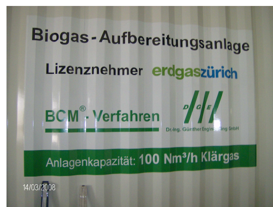
First biomethane plant in container design for the Erdgas Zürich AG
